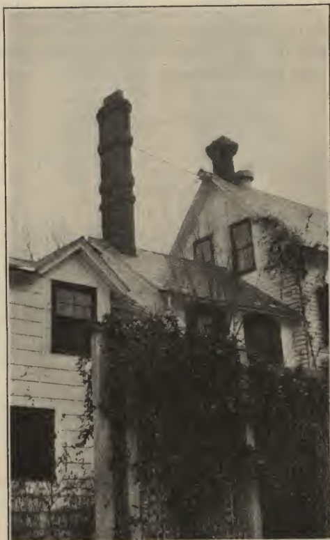
FIG. 3.—Extensions to the chimney required in order that it might draw properly.
